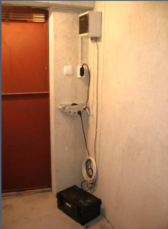
ETNA unit in the basement
