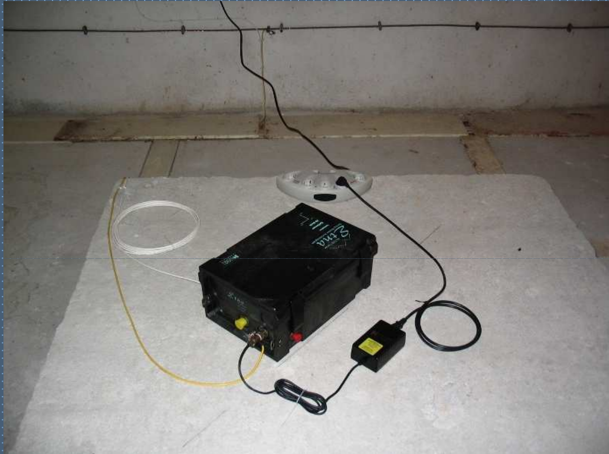
Typical installation ETNA 4498 (Krupnik station) SW Bulgaria
